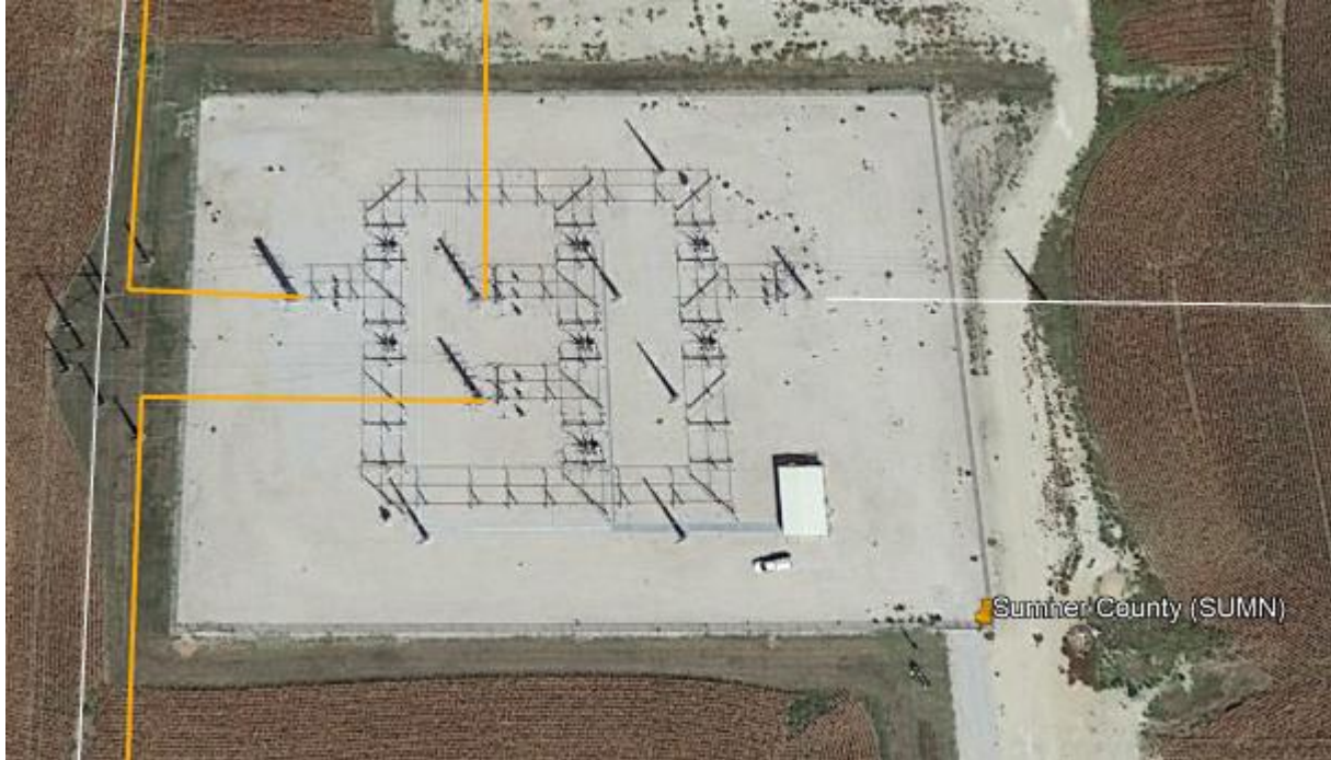
Figure 32 – Sumner County 138kV Substation
